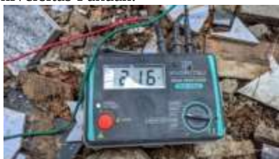
Gambar 8. Hasil pengukuran pentanahan area lift masjid
